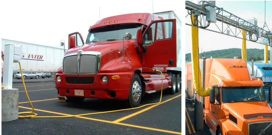
Figure 34: Examples of Truck Stop Electrification
