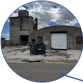
1. Deteriorated or Deteriorating Structures
