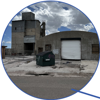
1. Deteriorated or Deteriorating Structures
