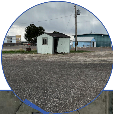
1. Deteriorated or Deteriorating Structures
