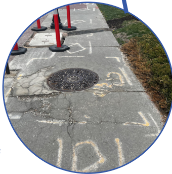
5. Deterioration of Site or Other Improvements
