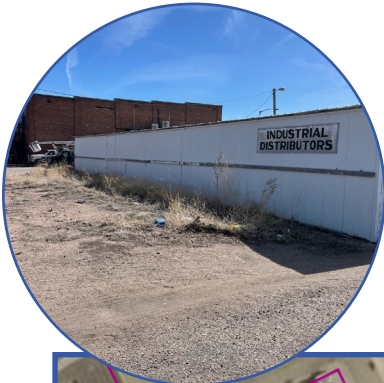
1. Deteriorated or Deteriorating Structures
