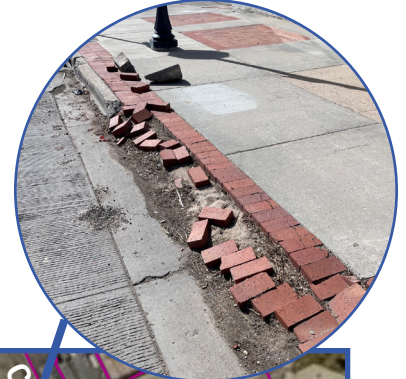
3. Deterioration of Site or Other Improvements
