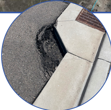
5. Deterioration of Site or Other Improvements
